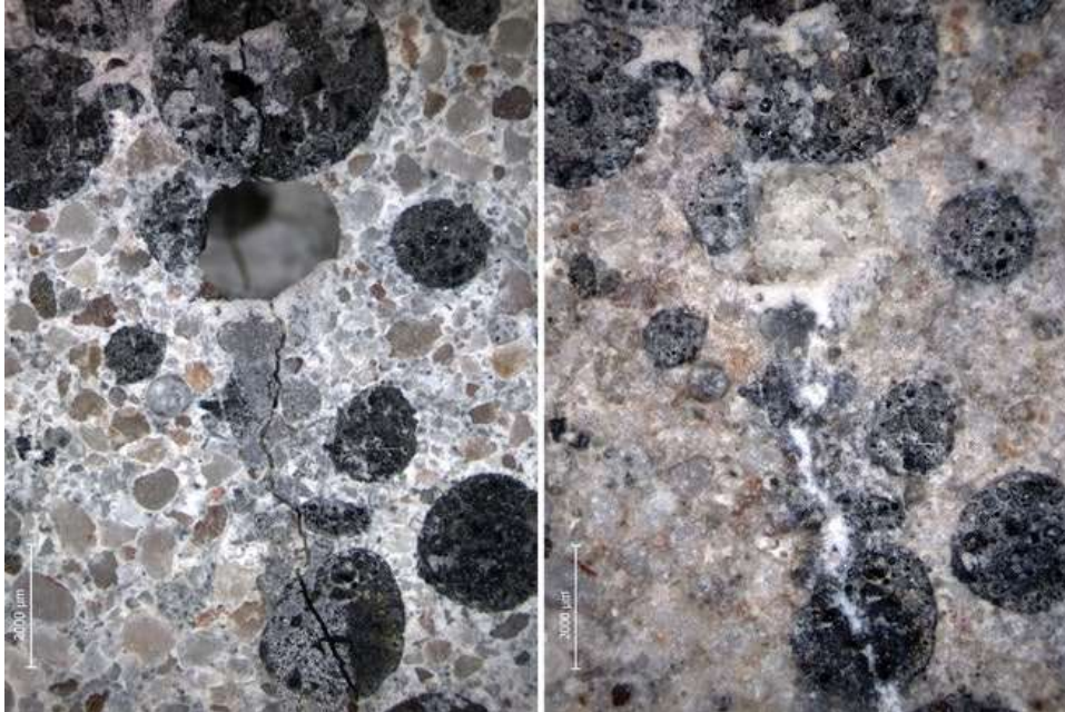
Cracked bio-concrete before healing (left) and after healing (right)
